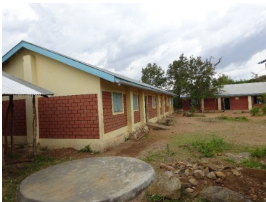
Foundation and gutters installed by Giribe Primary School (above) are ready for tank installation.
